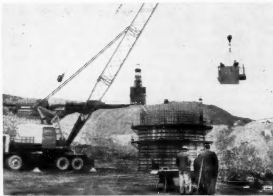
TUOLUMNE shaft will be a central pumping station. Waste from the Berkeley pit will be dumped around concrete tower.
